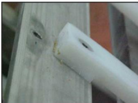
Avoid overlapping materials where joints cannot be sealed, creating harborage opportunities.
