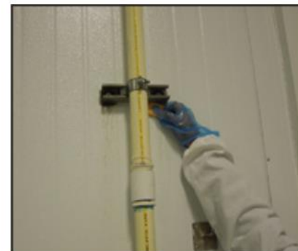
Condensation on walls, ceilings and behind pipes and conduit has been shown to promote Listeria establishment in the facility. Dripping to a concrete berm at the floor, especially if poorly grouted and sealed, can lead to intrusion of insulation and become a long-term reservoir for periodic contamination.
